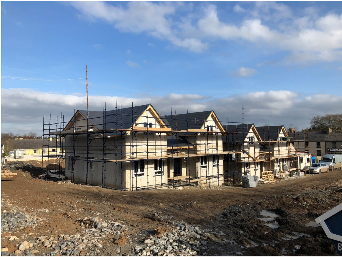
Photograph 1 – House numbers 1 – 4 incl. Roofing complete, internal fit out commenced. External wall insulation being installed.
